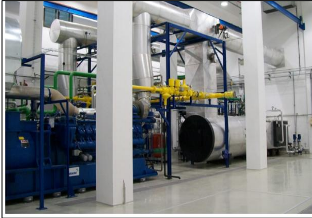
Figure 2. Trigeneration Power Plant
